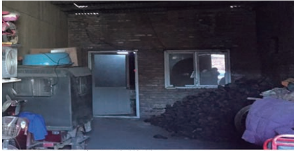
Coal-fired boiler before renovation
