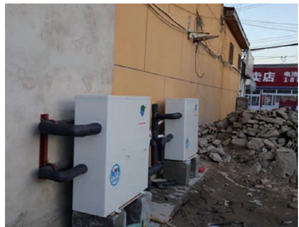
The host heat pump after transformation (installed outdoors)
