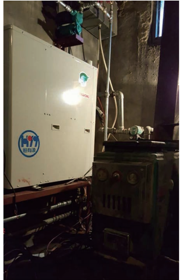
The host heat pump after transformation (installed in original boiler room)
